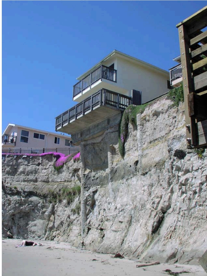
Seacliff erosion in the Isla Vista area of Santa Barbara has undermined this student apartment.
