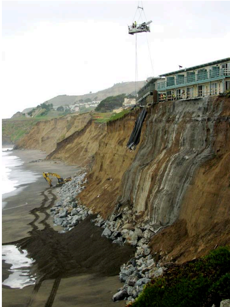
January 2010 Emergency cliff stabilization in progress in attempt to protect apartments in Pacifica.
