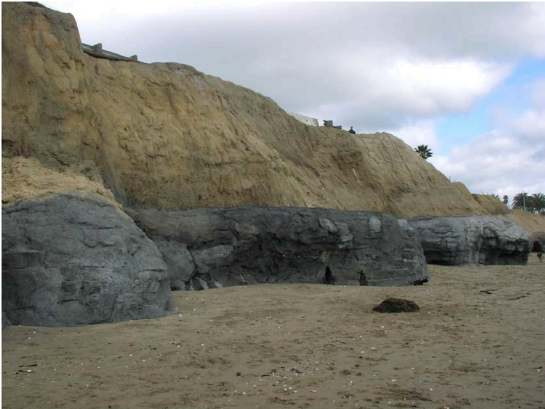
A soil nail wall consisting of shotcrete or gunite textured and colored to match the natural rock was used to stabilize the cliffs along Pleasure Point.
