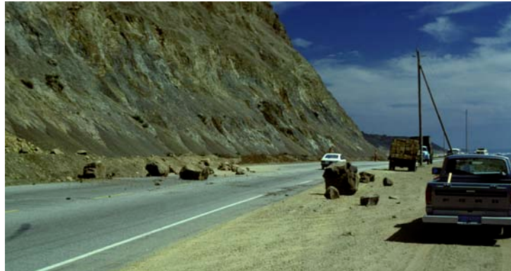
This 1978 photograph shows one of the rock falls on Highway One at Waddell Bluffs that made it through the trench that was designed to catch the rocks.
